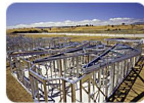
Steel framing has the highest strength-to-weight ratio of any construction material, which means less material is required to carry the same structural loads.
